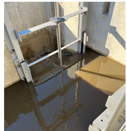
Clarifier Flow Splitter in Operation
